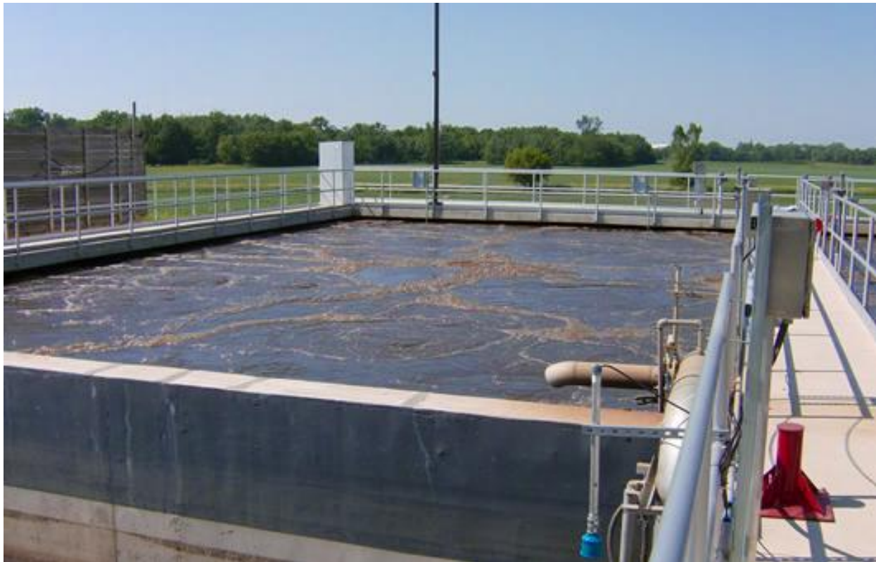
Figure 10-13: Aerobic Digester (Courtesy of APG Neuros)
