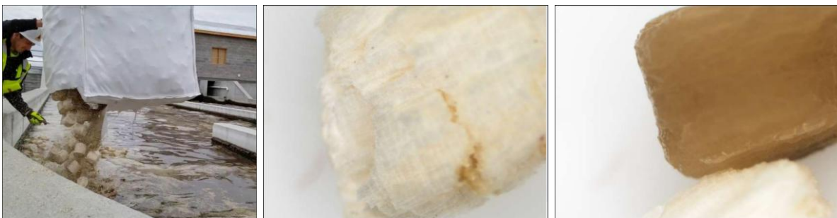
Figure 10-10: MOB Media Installation and Biofilm Growth on Media (Courtesy of Nuvoda)
