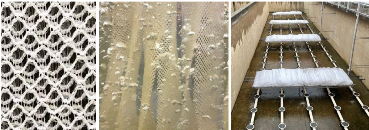
Figure 10-9: Fixed Media and Installation Example (Courtesy of Entex)
