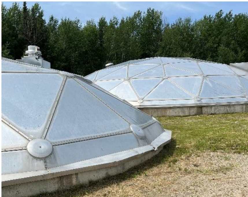
Figure 10-2: Existing CTUs at the Sioux Lookout WWTP
